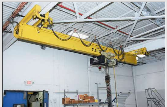
Yale 7.5-Ton Bridge Crane
