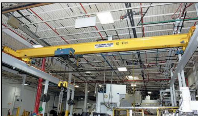
Mt. Clemens 10-Ton Overhead Bridge Crane
